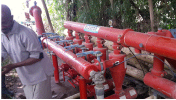
Figure 3. Large electric pump in Kobo-Girana, North Wollo
